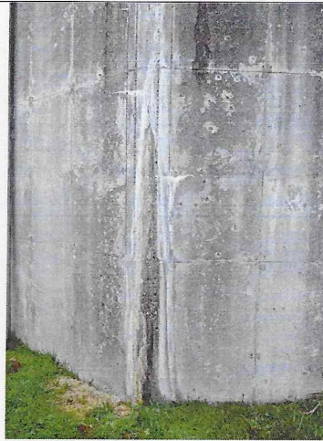
Tank corner with cracks
