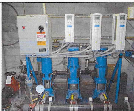
Booster pump station and VFDs.
