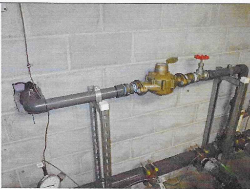
Source meter? (in pump house)
