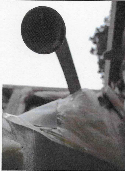
Screened well vent
