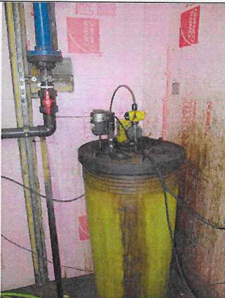
KMnO4 feed tank and injection pump
